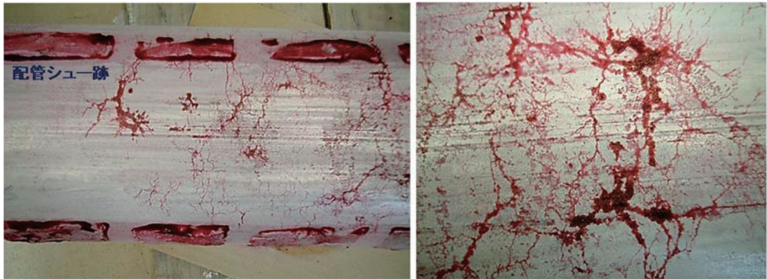
図1.8 Damage cases of ESCC under high stress environment in between the support shoe and the longitudinal welding of pipes
