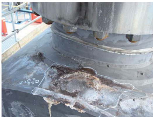
Rainwater penetration with pitting regions from the clearance of equipment M / H
